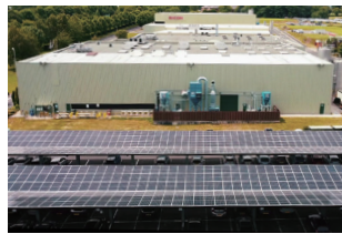
Private power generating equipment at a RE100 certified British plant
