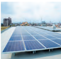
Solar panels at Gifu Branch
