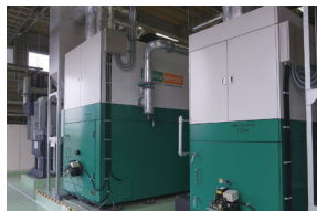
Wood biomass boiler
