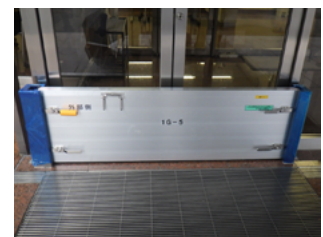
Installation example of water gate barrier at Ricoh Ikeda Plant
