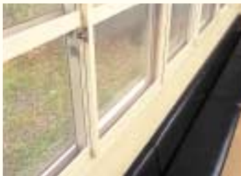
Double windows with a resin window frame
