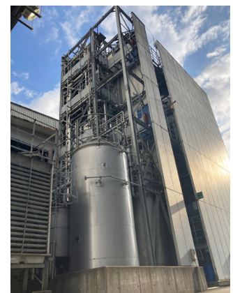
Facilities that conduct reusing of solvents (distillation facilities)
