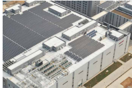
Photo 2: Solar panels installed on the roof
