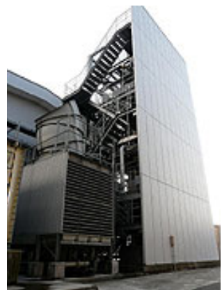
Facilities that conduct closed-loop recycling of solvents (distillation facilities)
