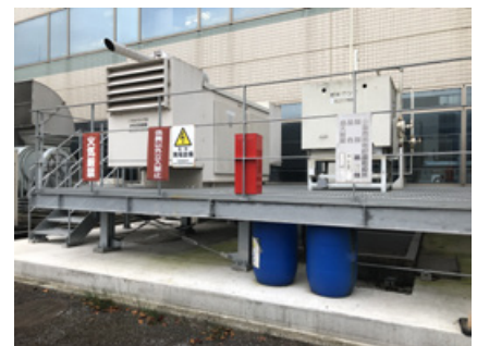
Emergency generator raised off ground (RTC)
