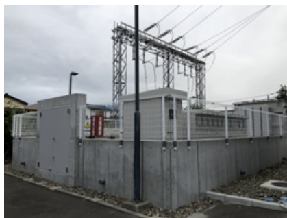
Extra high voltage substation; retaining walls (RTC)
